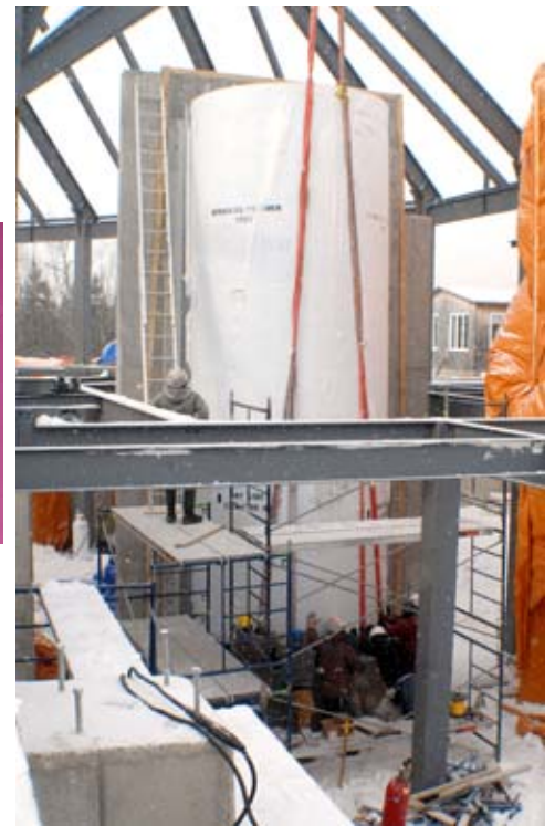
The new tidal display tank is hoisted into place at the Fundy Discovery Aquarium.
