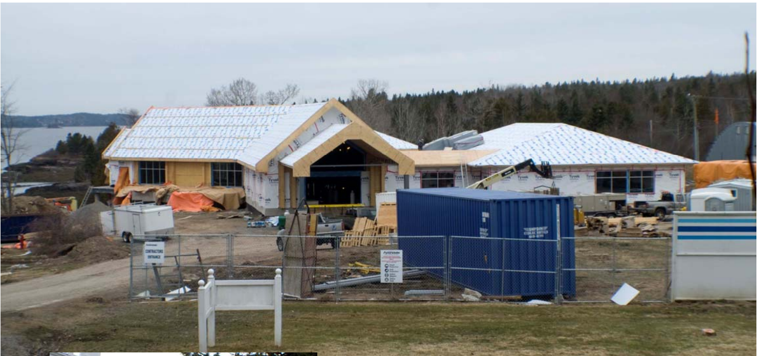
Above: The new Fundy Discovery Aquarium under construction. Now that the building itself is in place, the view seems to change on an almost daily basis as the summer 2011 opening looms.
